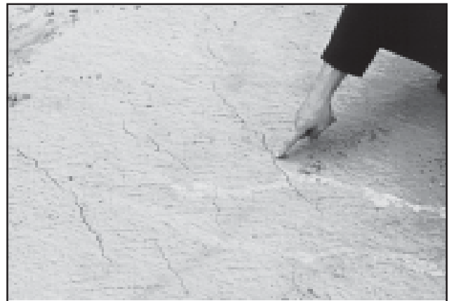
Plastic Shrinkage Cracks
