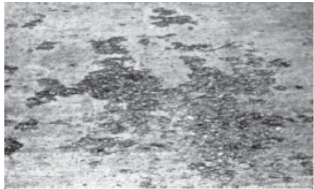
Scaling concrete surface
